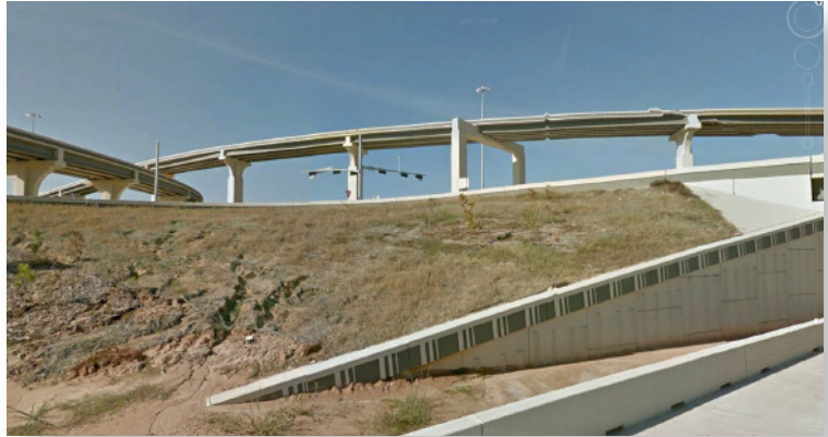
Significant rilling and lack of vegetation was common in the project area. March, 2018.
